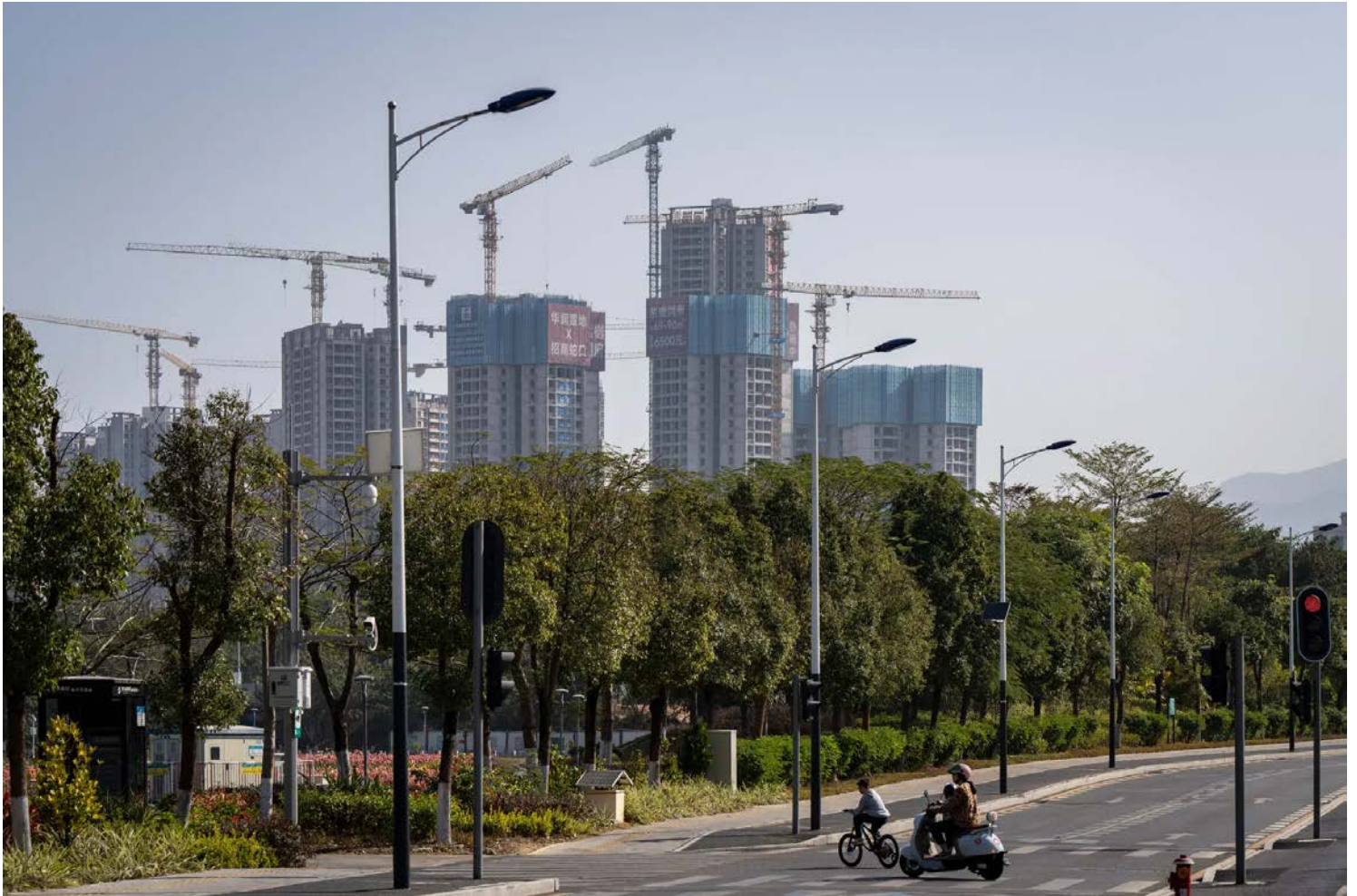
New apartment construction in Shenzhen in January. Qilai Shen for The New York Times
