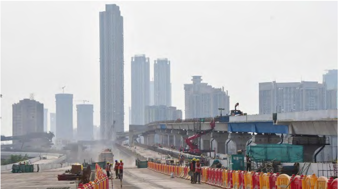
A view of ongoing road construction at Sewri in Mumbai - Bhushan Koyande/Hindustan Times/Getty Images
